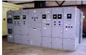
480VAC Generator Control switchgear built for Pemex
